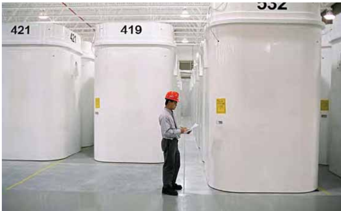
Used fuel dry storage containers
