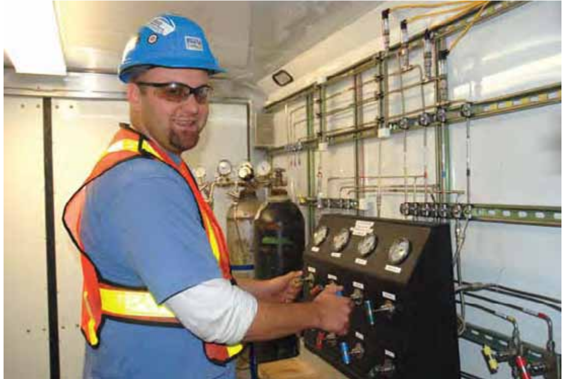
Borehole hydraulic testing trailer
